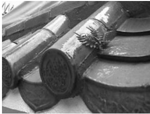
Photo above author's own: a close-up of the Shiwan tiles at the same temple, old mixed with new tiles.
